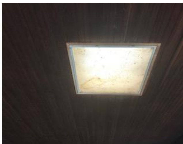
Entrance lighting before changes.
