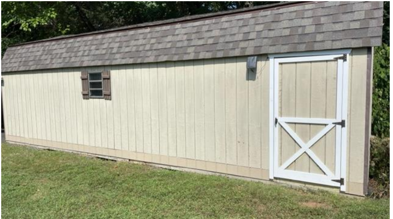
Shed with rotted wood and door replaced.
