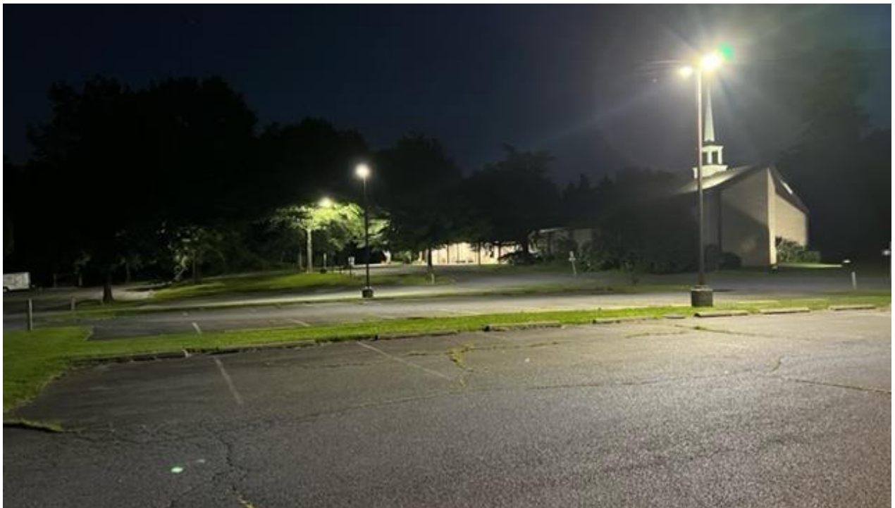
Church Parking Lot with new lighting.
