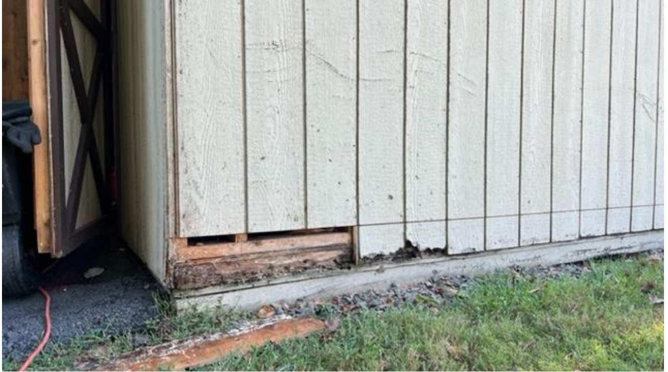
Shed showing rotted wood.
